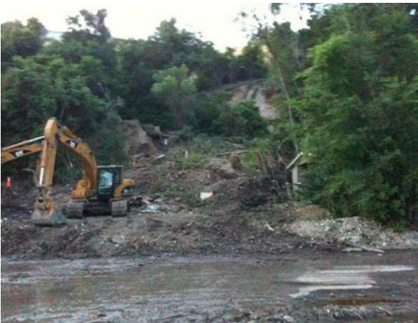
Above: July 2009 – Canyon Road Mudslide and Canal Failure Right: Mt Logan Stake Volunteers working to remove the debris.
